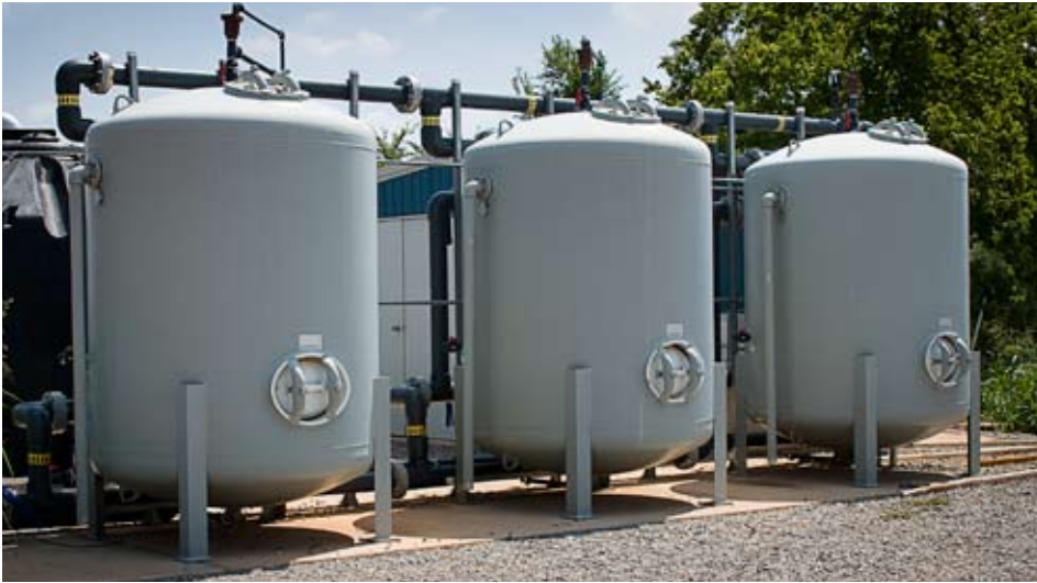
The three arsenic removal vessels at the Norman site. Three vessels are required to provide series flow and redundancy to the system
